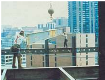
At-risk workers without appropriate safety equipment
